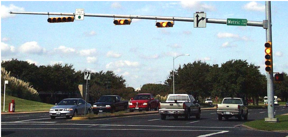
Figure 2.1 Typical Traffic Signal Mast-Arm (Koenigs et al., 2003)
