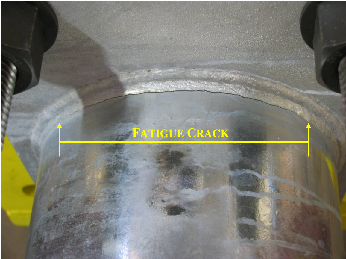
Figure 4.3 Fatigue Crack Propagation at Specified Point of Failure
