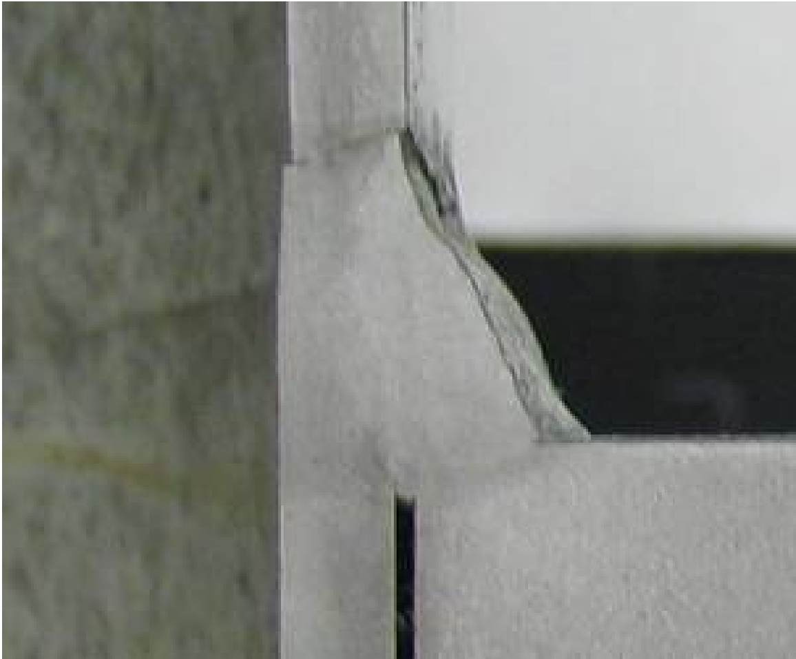
Figure 6.4 Detailed View of Etched Failure Location
